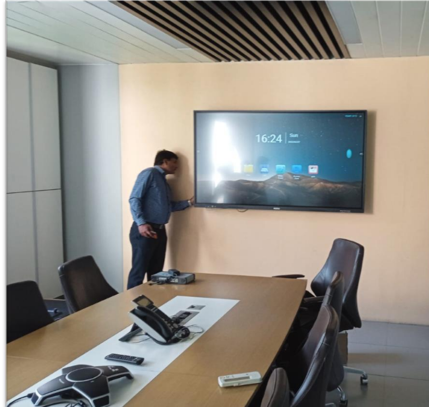
75" Inches Interactive Display Installed at Rohan Builders, Shivaji Nagar - Pune
