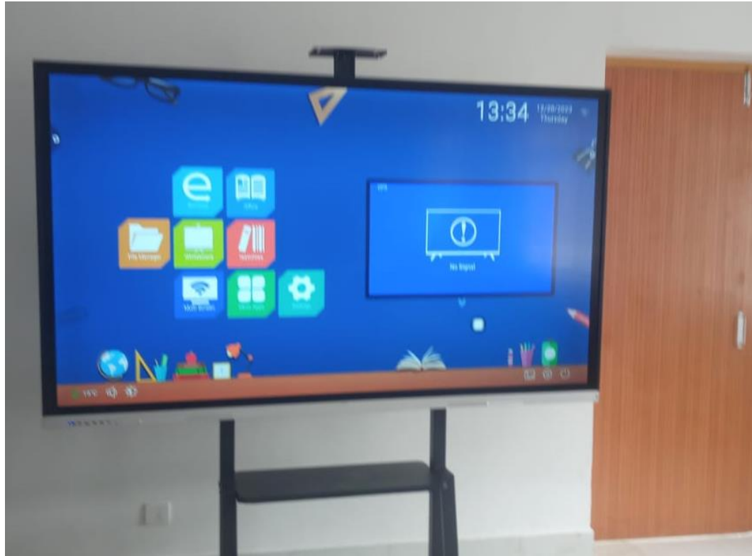
2 NO.S 86" Inches Interactive Display Installed at Government Of Electronics & Information Technology , Sikkim
