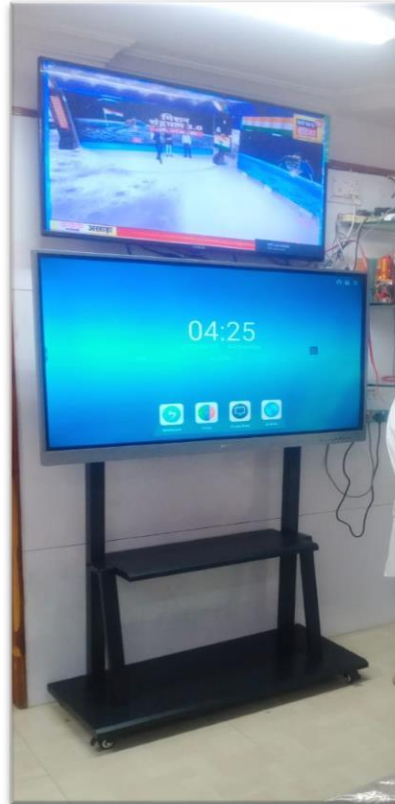
55" Inches Interactive Display Installed at Branhma Kumaris, Mount Abu
