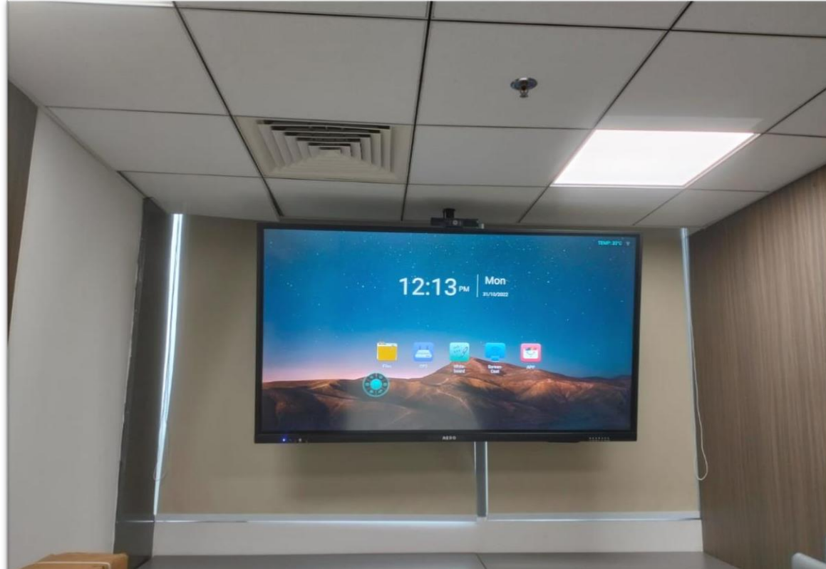
75" Inches Interactive Display Installed at Bliss Anand, Sikanderpur
