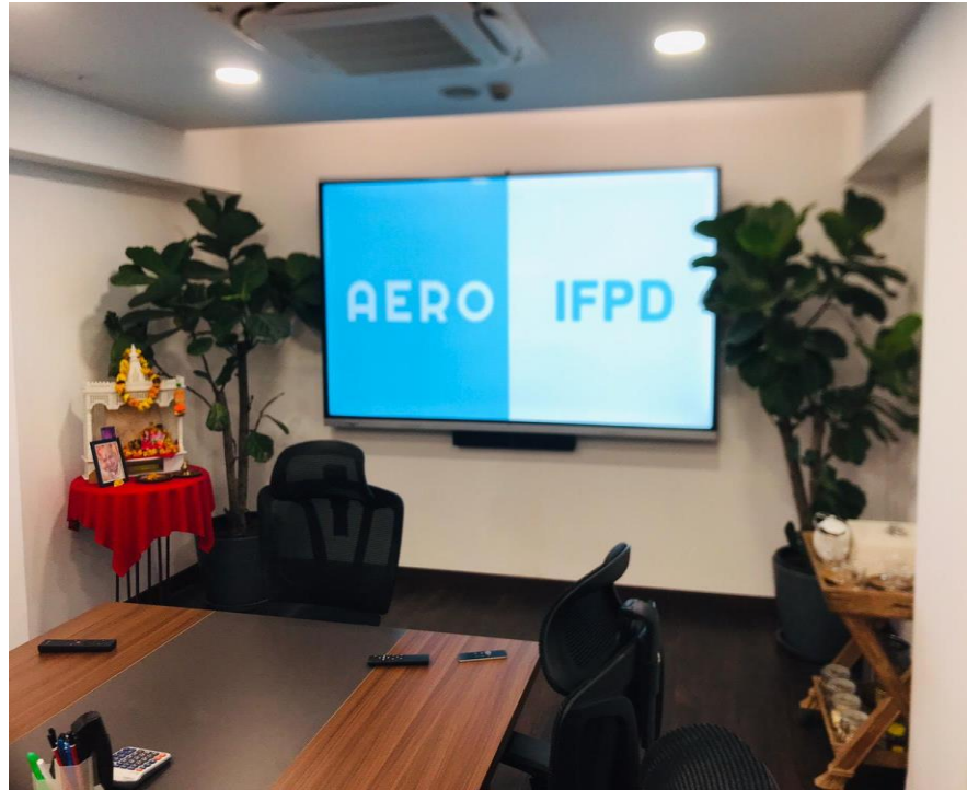
86" Inches AIFP Installed at Abesit Noida- Delhi
