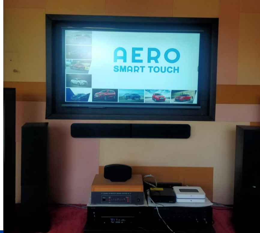
55" Inches Interactive Display Installed at Sound Lounge, Arjangarh - Delhi
