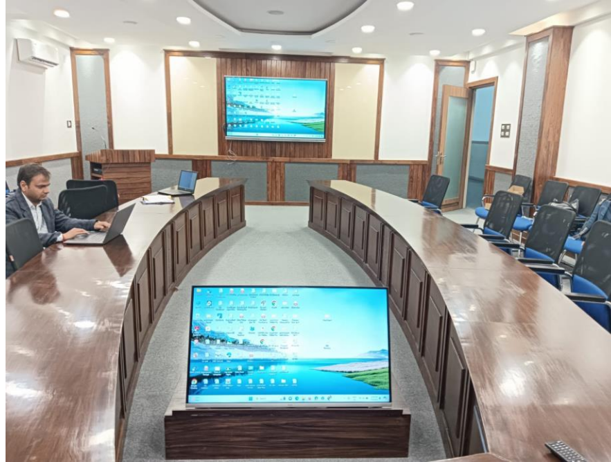
98" Inches AIFP Camera & Mic Installed at Mechtech Udyog Vihar - Delhi
