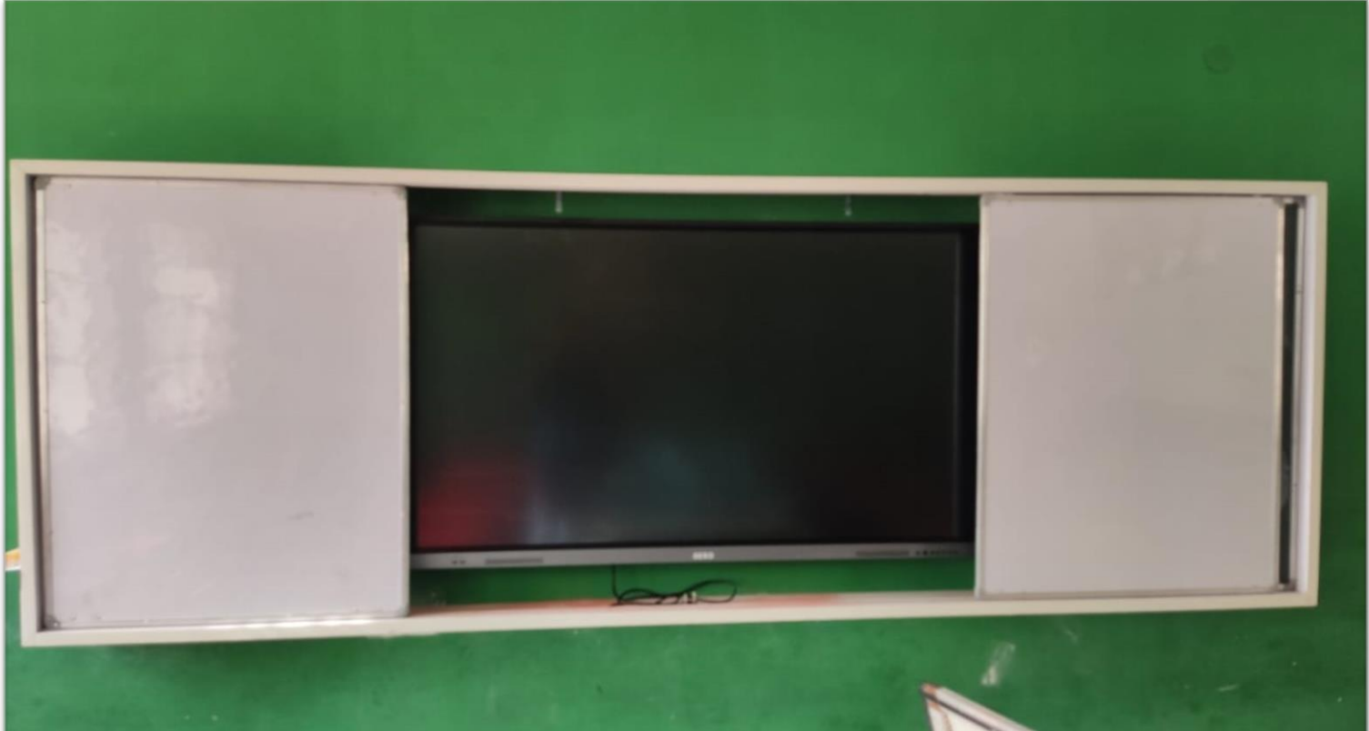
65" Inches Interactive Display Installed at Kendriya Vidyalaya, Mohali
