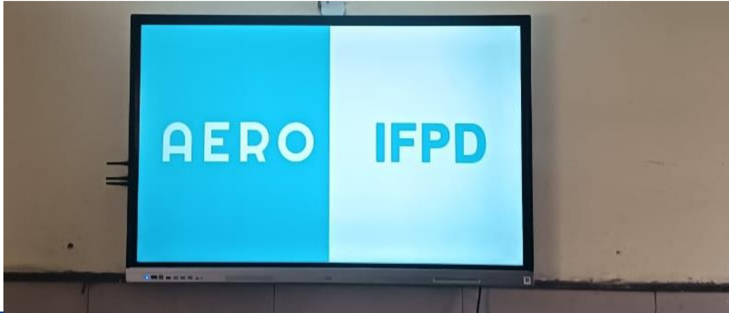
55" Inches Interactive Display Installed at Government School, Rani Bagh - Delhi
