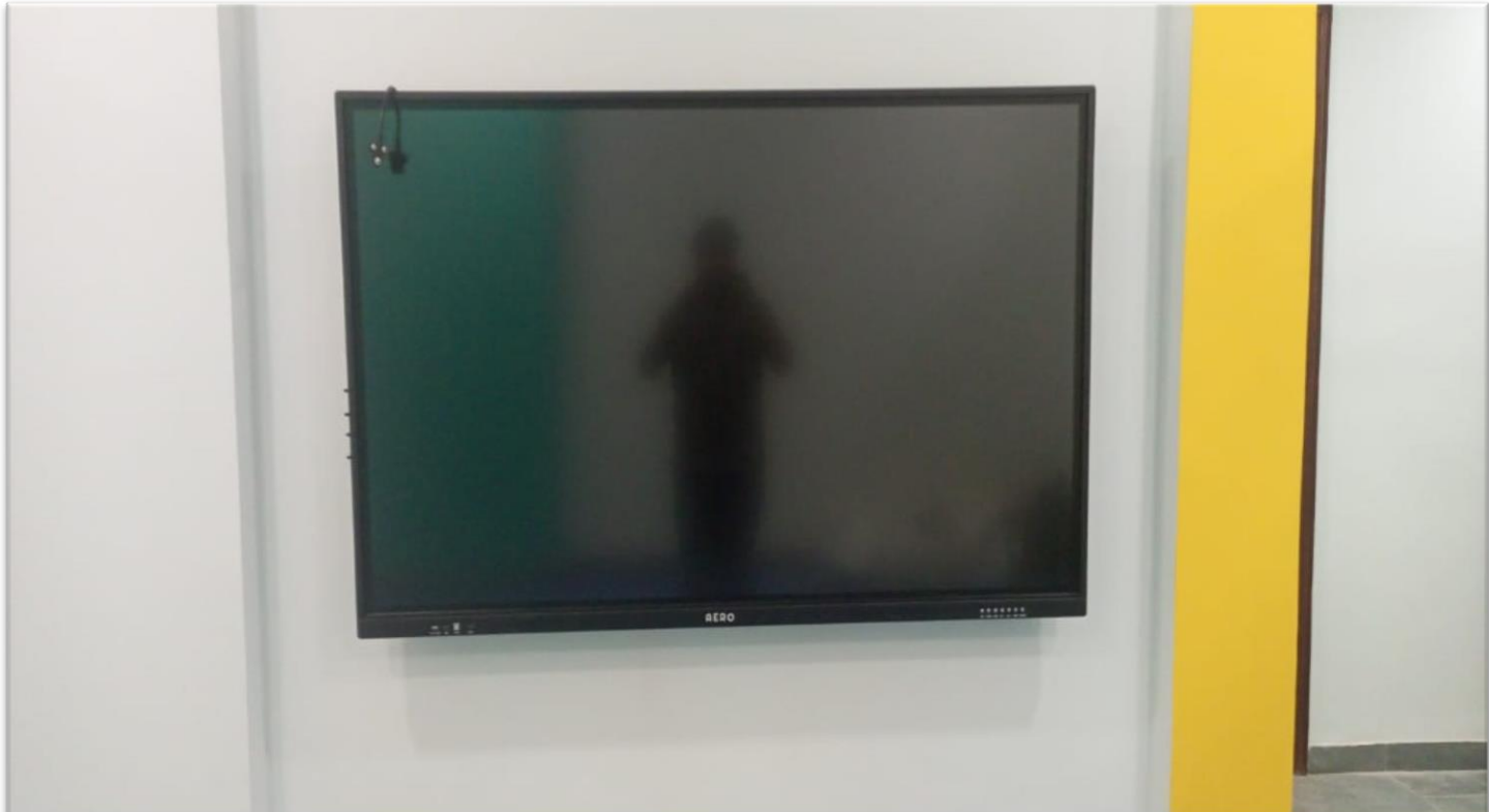
65" Inches Interactive Display Installed at New Children's Academy, Ghaziabad
