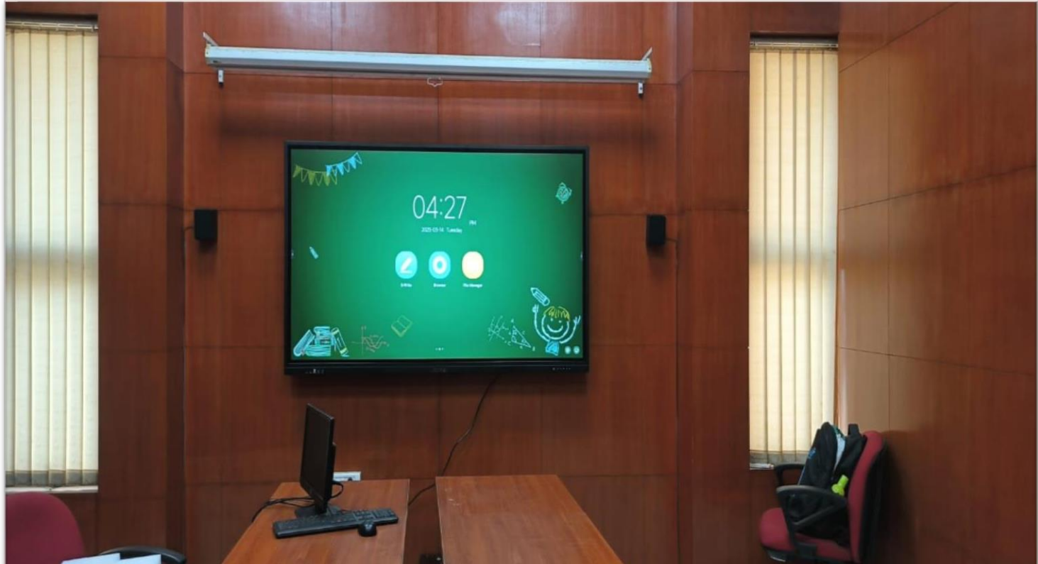
75" Inches Interactive Display Installed at ONGC, Raigarh
